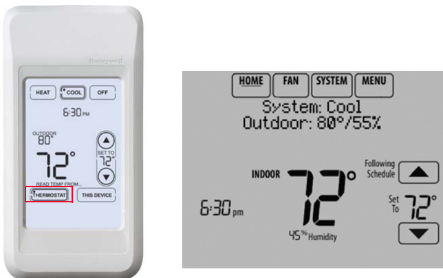
Fig. 302. Reading temperature at the thermostat.
