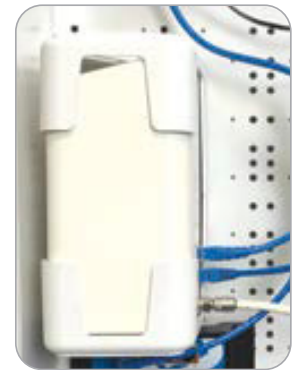
Installed in SOHO Pro media panel
