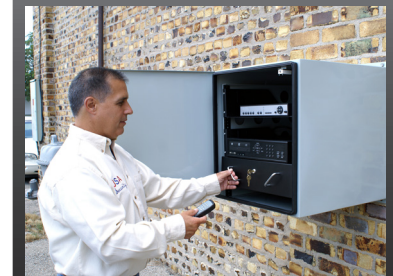
Rack Enclosure mounted on a wall
