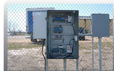
Along a gate using metal tubing to run wiring from one enclosure to another
