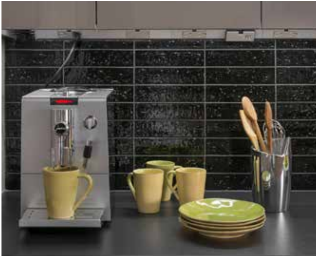
Under-Cabinet Lighting System installed in a kitchen.
